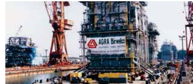
4 Modules Pyrolysis Furnace Client : AGRA Birwelco ExxonMobil
