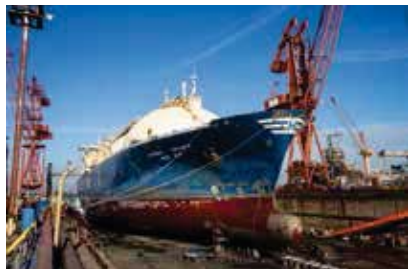
LNG Carrier Hyundai Aquapia Dry docking and repair Client : Hyundai Ocean Service Co Ltd Weight : 77,564 dwt
