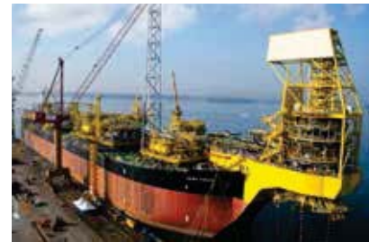
FPSO Kikeh Conversion of a tanker to an FPSO for Malaysia's first deepwater field Client : MISC Berhad / SBM Location : Offshore Sabah, East Malaysia
